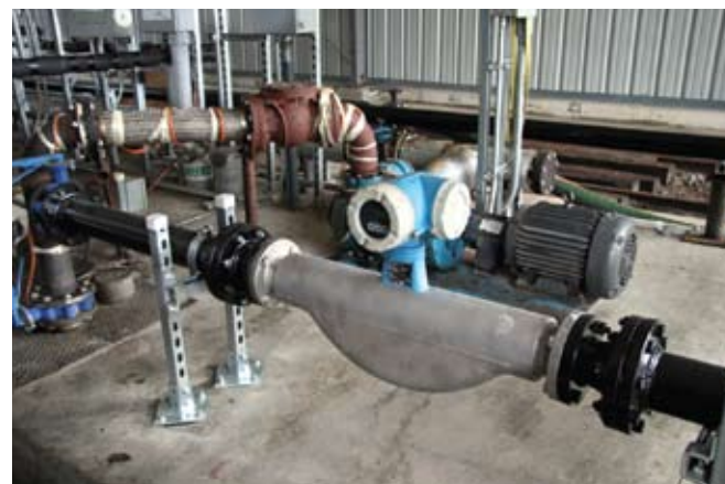
An Endress+Hauser coriolis meter is used for precise metering of transload cargoes at the Morristown location.
