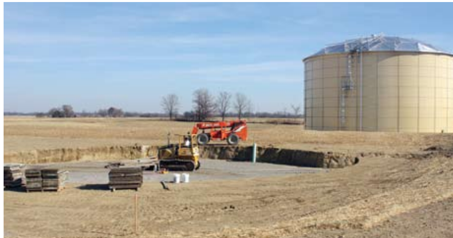
Work is underway on a second storage tank at the Morrystown IN transload facility. Additional space is available for two more storage tanks at this time.
