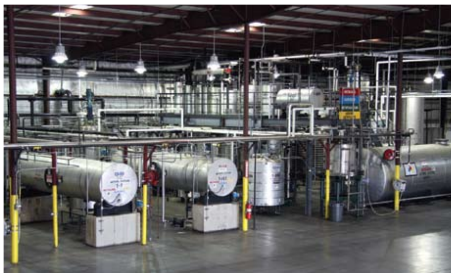
A subsidiary of Grammer Industries, Integrity Biofuels has a capacity to produce 10 million gallons of biodiesel a year from soybean oil. The Morrystown IN transload facility operates under the Integrity Biofuels name and shares space and resources with the plant.
