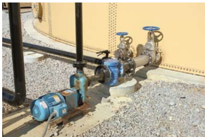
An electrically powered pump from MP Pump Inc is used to transfer product to and from the storage tank at the Morristown site.
