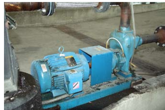
Electrically powered pumps from MP Pumps Inc are used to transfer product at the Grammer Industries transload sites.
