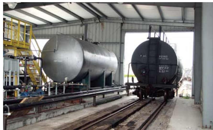
At Morristown IN, product transfer to and from rail tankcars and tank trailers is performed in a covered area that provides plenty of protection from the weather.
