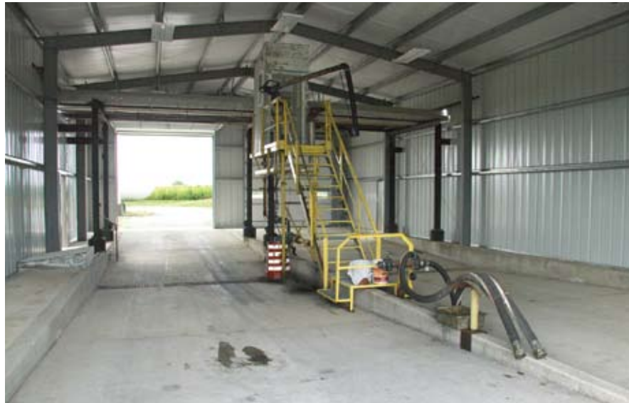
This two-bay enclosed loading rack was a recent upgrade for the Van Wert OH transload terminal. The enclosure provides a safer and more comfortable work area during bad weather.
