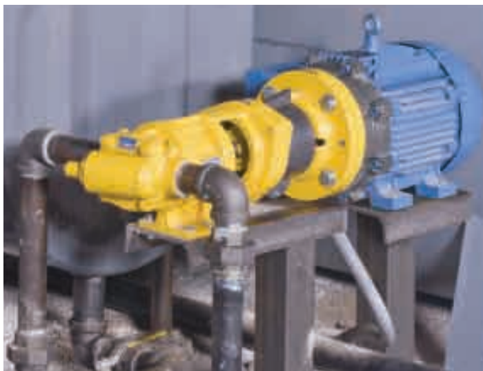
ProVane pumps are used for methanol recovery, caustic, magnesol and tallow/soy oil transfer applications in the above facility
