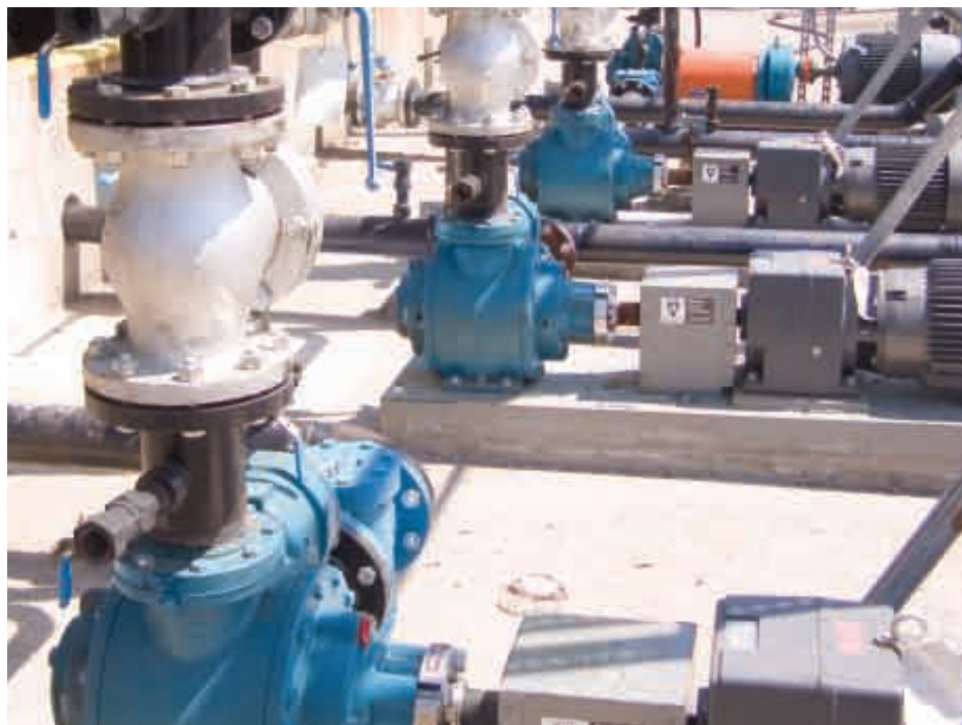
Blackmer sliding vane pumps in use at one of the largest biodiesel production facilities in the US
