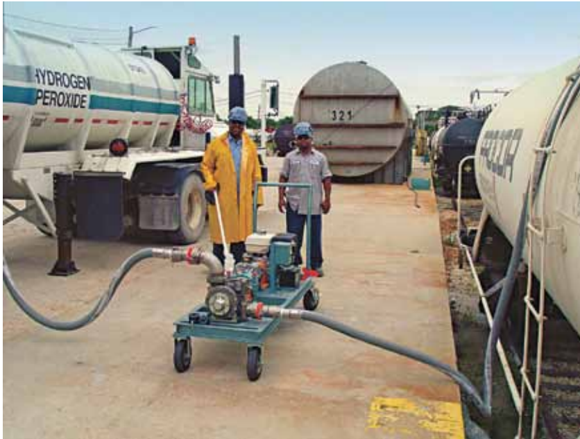
Operators at this chemical distribution/storage terminal facility transload hydrogen peroxide from a railcar to a transport via a sliding vane pump.
