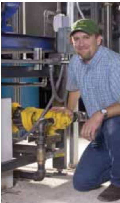
Figure 1. Scott Johnson, president of GEN-X Energy Group, kneels next to one of the many Blackmer ProVane motor speed sliding vane pumps located in the plant.
