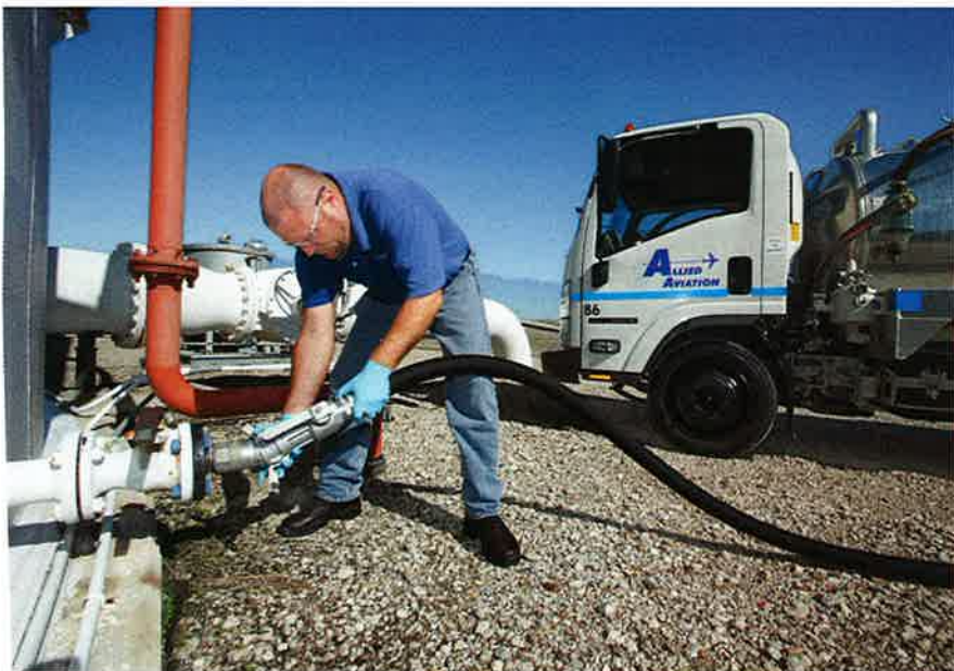
Steve Minter attaches a vacuum hose to one of 200 service points on the hydrant-style fuel distribution system at IAH. The system gets a monthly routine service inspection from the Allied Aviation maintenance team.
