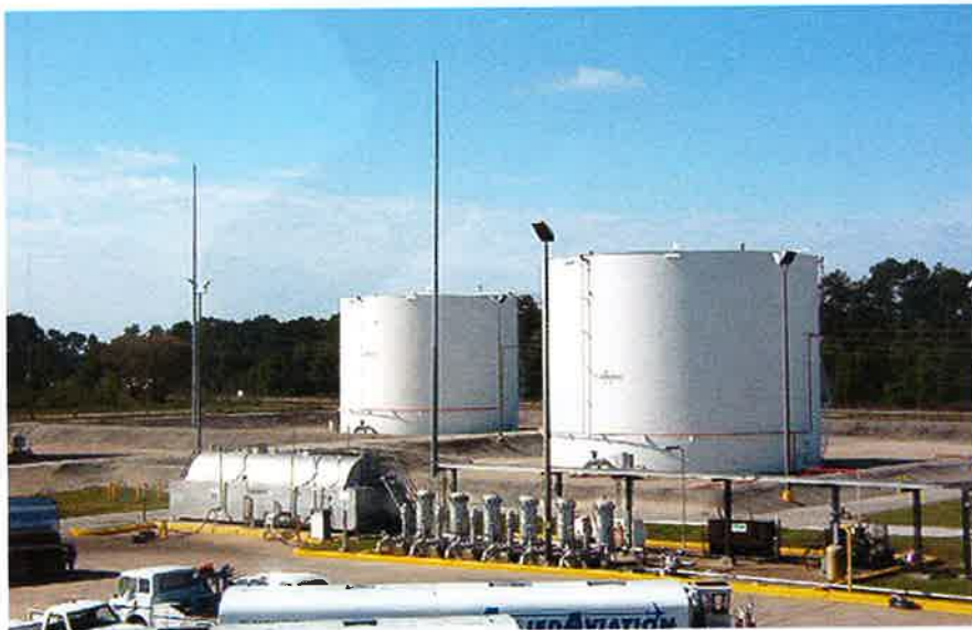
Fuel storage at IAH totals 13 million gallons—all of it Jet A—in 10 aboveground tanks. The tank farm and the hydrant-style distribution system to the IAH terminals is managed and maintained by Allied Aviation.
