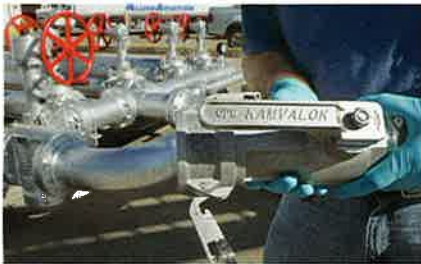
OPW's Kamvalok dry disconnect couplers make the process of servicing the fueling hydrant system at IAH safer for maintenance personnel and the environment.
