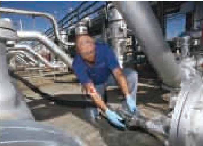
The hydrant system, which consists of more than 200 service points, is serviced once a month
