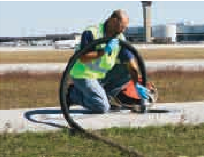
The hydrant system has over 200 service points
