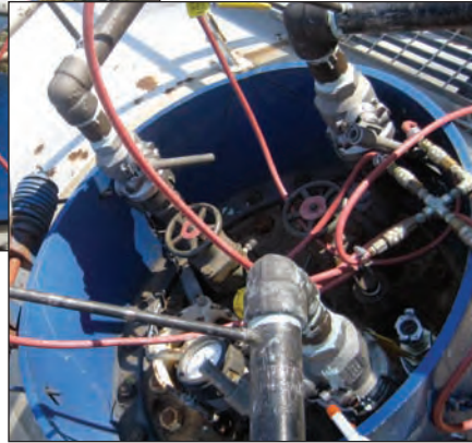
OPW Drylok™ couplers equipped on the butadiene railcars allowed for a faster, safer and efficient transfer during the evacuation process.
