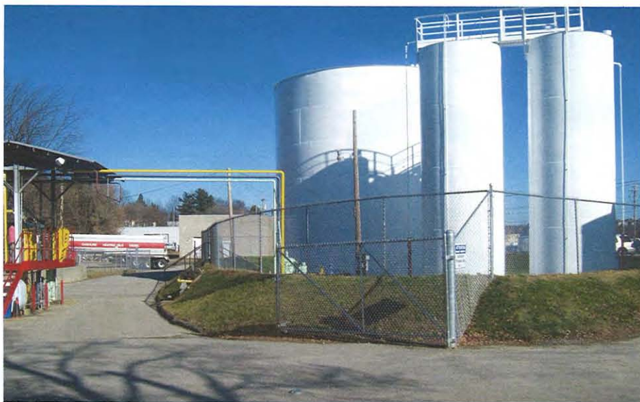
OPW's automated tank gauging system has helped Dead River expand its services to customers
