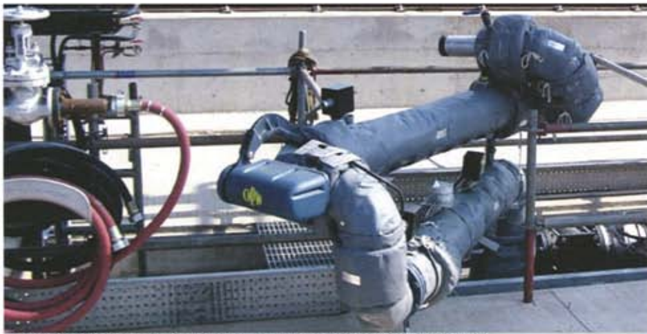
When converting to bottom loading, rack layout needs to be reconsidered
